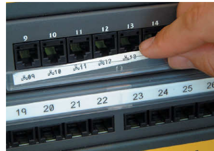
Punch block & patch panel labels
