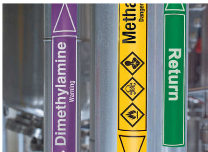
Pipe & valve marking
