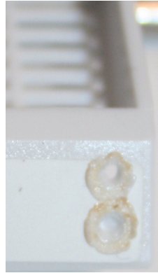
Rivet Appearance with accumulated Residue
