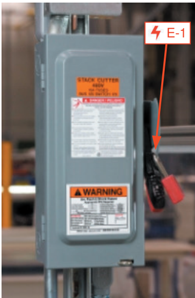
Disconnect in Engine Room - West of Machine
