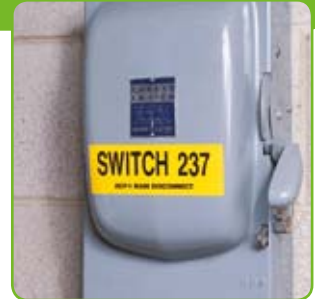
Panel & Switch I.D.
