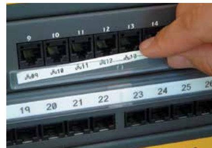
Punch block & patch panel labels
