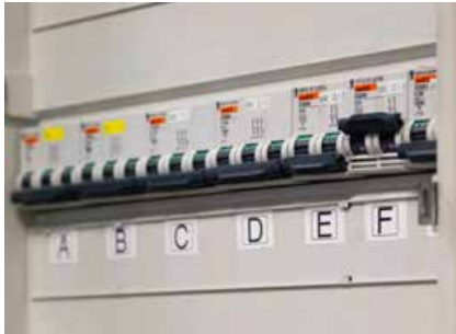
Circuit breaker marking
