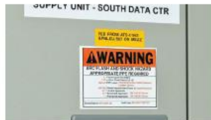
Arc Flash Services and Labeling
