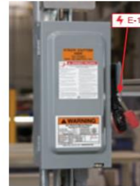
Disconnect in Engine Room - West of Machine
