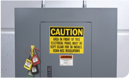
Panel and Enclosure ID
