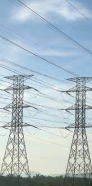
220kV Transmission Tower
