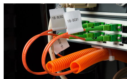
Fiber Optic Cable Markers
